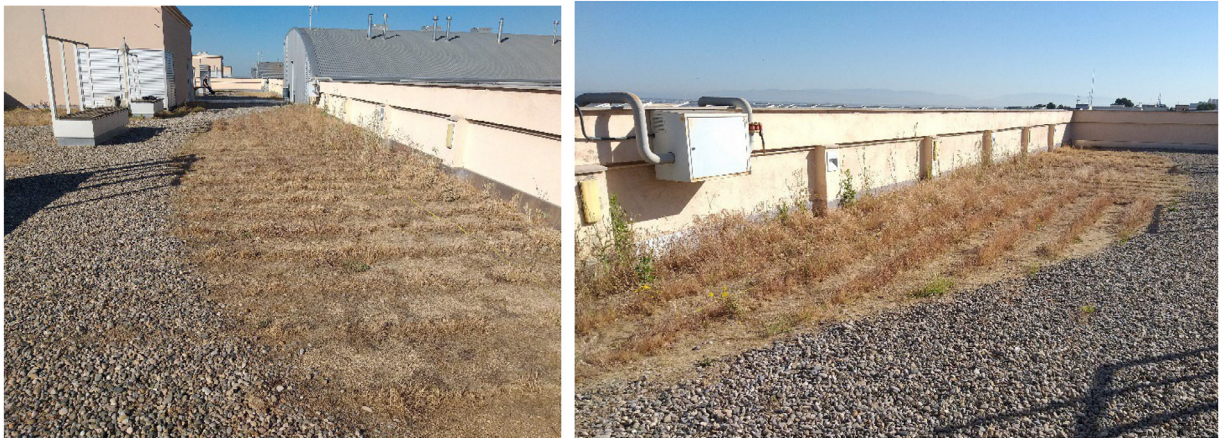
Fig. 5. “H buildings” at the Lleida Agri-food Science and Technology Park (PCiTAL) Lleida, Spain. Example of a green roof in operation but not receiving the expected benefits.
